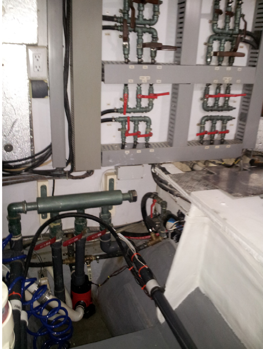
Pictured Above: Fuel valve selector switches (upper right), and 3-way PVC outflow bilge emergency crash pump (w mesh strainer) connected directly to diesel CAT engines. All handles labeled and in good condition.
